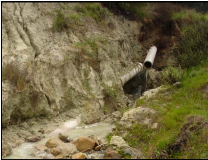
2010 Storm Damage - Line Break at the Trabuco Canyon Road Switchbacks
