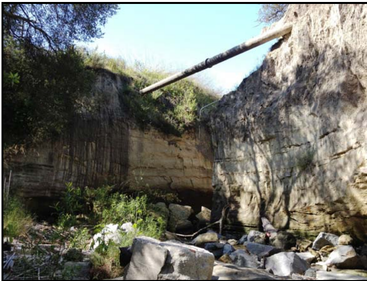
The damaging effects from the 2010 Storm Event on TCWD's Raw Water Transmission Line.
