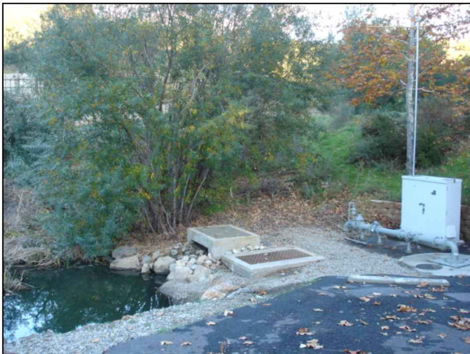
Figure 4.5 Tick Creek Pump Station
