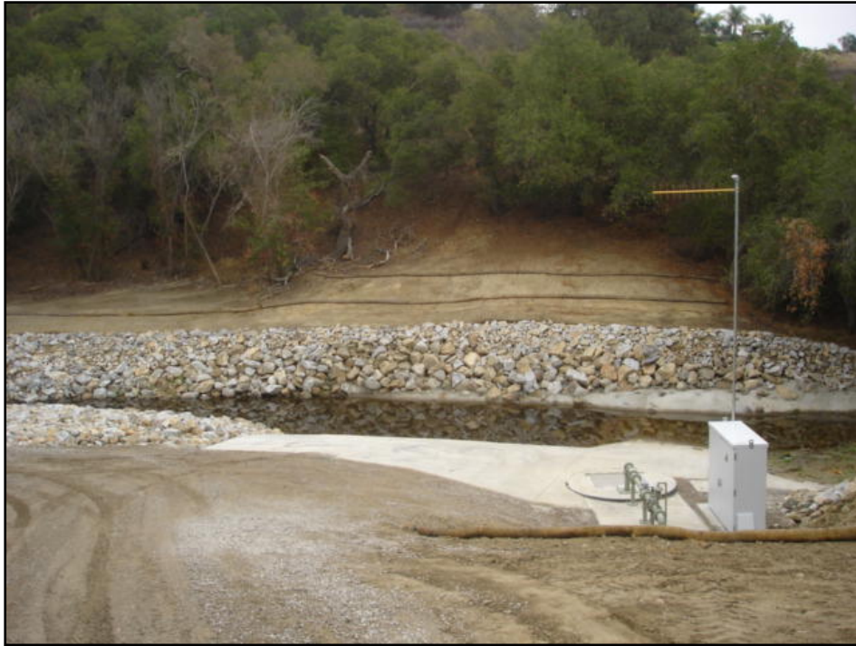
Figure 4.4 Dove Creek Pump Station
